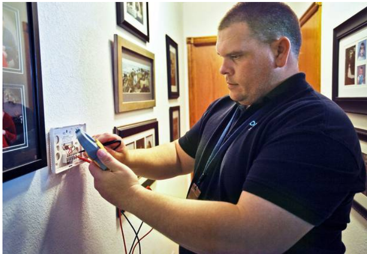
Oklahoma Gas and Electric Co. worker Greg Henderson installs a new programmable thermostat Thursday at a house in Piedmont. The thermostat can communicate with a smart meter at the house to help reduce electricity costs. Photos by Chris Landsberger, The Oklahoman
